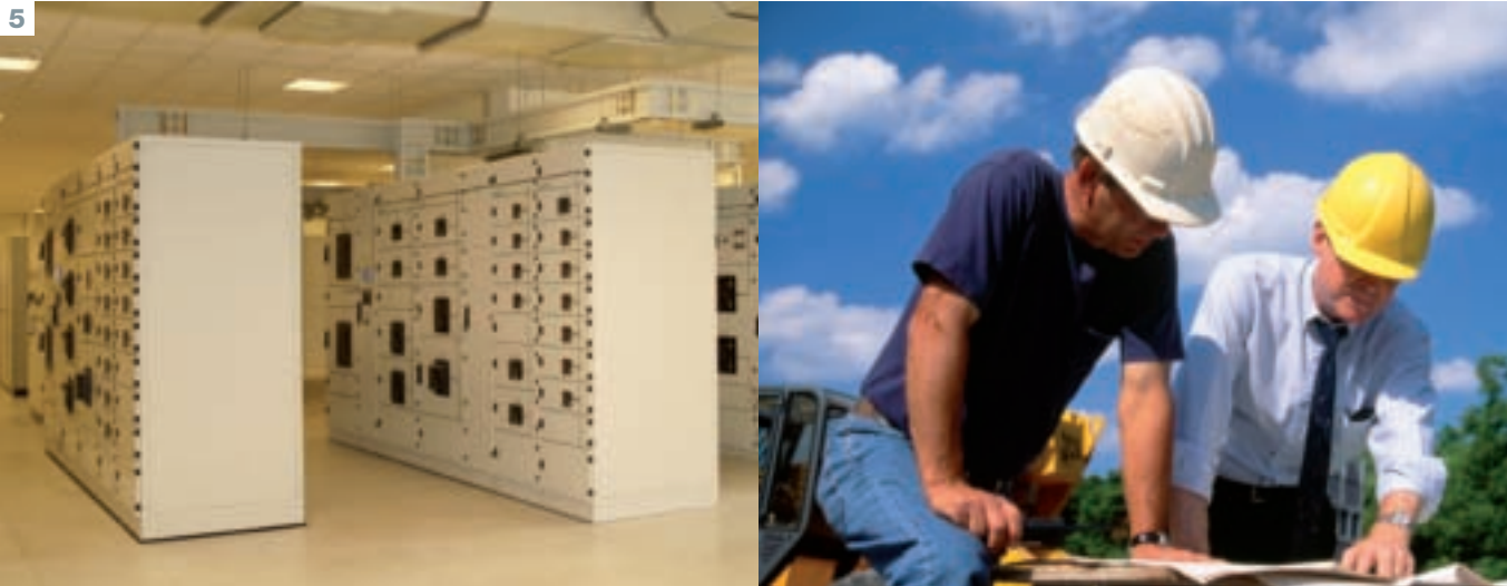
5 - Sala quadri / Electric panels room
